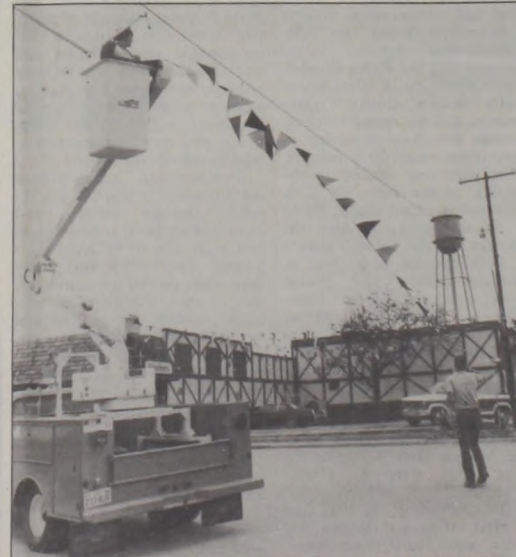
TWO TELEPHONE EMPLOYEES of Muenster Telephone Company attach strings of red, yellow and black pennants across Main Street in preparation for Germanfest. They are shown at work near Fischer's Meat Market.
