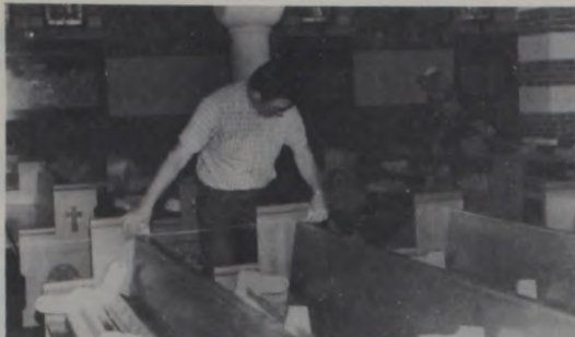
LEADING TOWARD the eagerly-awaited restoration of religious services in St. Peter's Church in Lindsay is progress indicated in these photos. Two weeks ago, Richard Neu, an employee of Joe Walter Lumber Co., was trimming carpet at a side altar. Last week, workers from the Wagoner Bros. Manufacturing Co. of Jonesboro, Ark. replaced the
