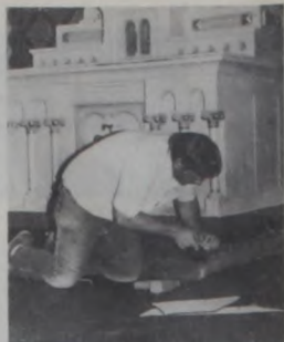
beautifully refinished pews. This week, other last minute finishing touches and clean-up are being carried out by Lindsay parishioners. On Palm Sunday, the 10 a.m. services will be celebrated in the church. The public is invited. The Saturday evening Mass and 8 a.m. Sunday Mass will be held in the Parish Hall.
