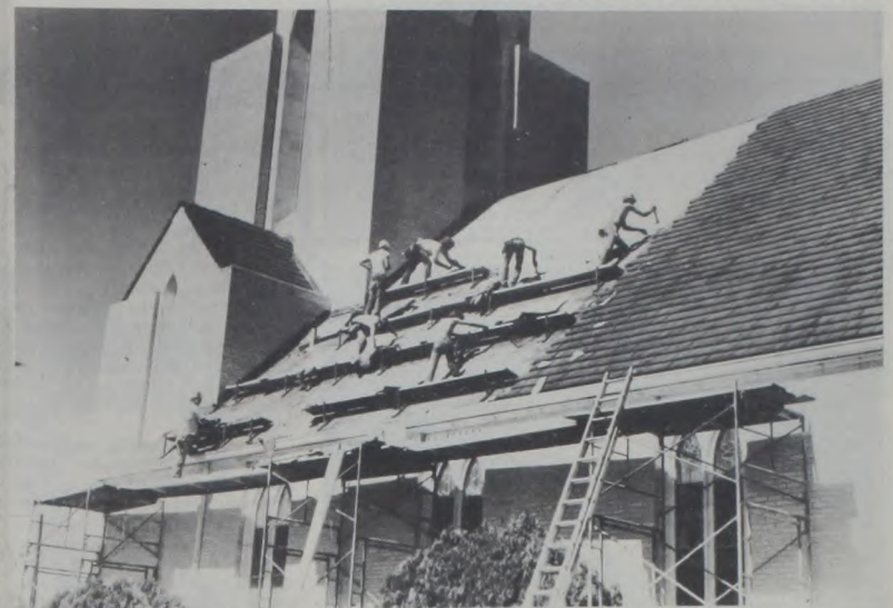
LIKE LOOKING UP to an ant hill, the view from ground level shows All Tile and Slate Co. workers dwarfed against the massiveness of Sacred Heart Church. They were agile and industrious in removing the old roof in preparation for the new. Dave Fette Photo
