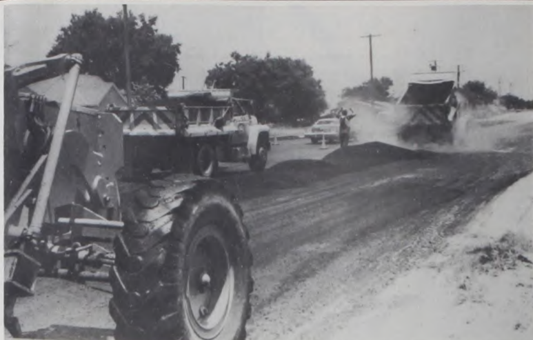
STATE HIGHWAY Department Maintenance crew gives North Main Street, from 7th to 9th, a new surface. Other bad places will be repaired, then the street will be sealed with oil and rock. Janie Hartman Photo
