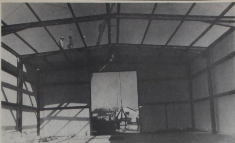
OUTSIDE WORK IS NOW COMPLETED on Gilbert Endres Distributor, Inc.'s new building. The 40' x 80' building will be used for truck maintenance and truck parking. A pit is in the floor of the building for easy working excess under the trucks. The insulated building can also be used for storage. Plans in the near future include enlarging the fenced-in yard behind the building. Janie Hartman Photo
