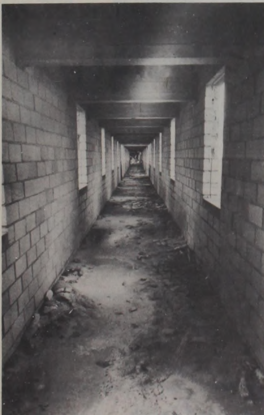
THE MAIN CORRIDOR of the hospital at Camp Howze, pictured above, once connected a 1,200-bed facility. Janie Hartman Photo
