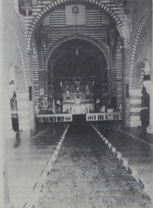
SAINT PETER'S CHURCH in Lindsay makes ready for interior redecorating. Pews have been removed and scaffolds are being erected. One rain-damaged area is visible in the upper right corner of photo. Sunday services will be held in the Parish Hall this weekend.
