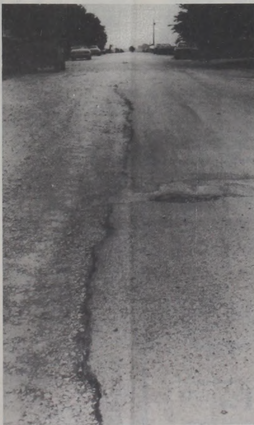
NORTH CEDAR STREET residents want the city to replace their street due to defective construction.
