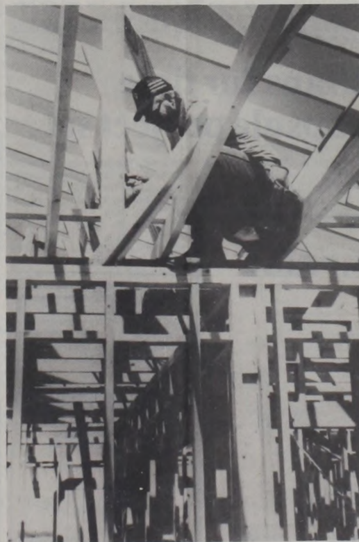
RUDY KOESLER , a carpenter at work on Dr. Gerald Graham's new dental office building, is shown as framework progresses at the location just south of his present office in the Medical Center. The new facility will have five operatories completely furnished including X-Ray equipment. In three rooms, large picture windows overlook the lake.
