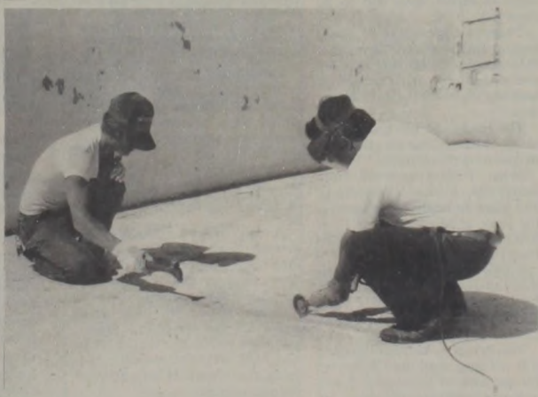
HAMMERING AND SANDING cracks in the bottom of the city swimming pool, David Dittfurth, left, and City Administrator Joe Fenton, right, ready the cracks for repairs. Once the old paint and loose concrete was hammered loose, a wire sander was used to clean the debris before the cracks were filled with a water-stop cement patching material. When that had dried a fresh coat of paint was applied to the floor and walls of the interior of the pool.
