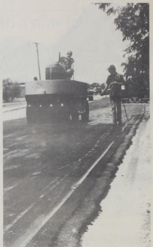
PAVING WORKERS for city street contractor Jones & Co. wet down the tires on a roller Monday to keep the asphalt from sticking in the summer heat. Just a little more paving remains to be completed in the city's massive street project this summer. Photo by Janie Hartman
