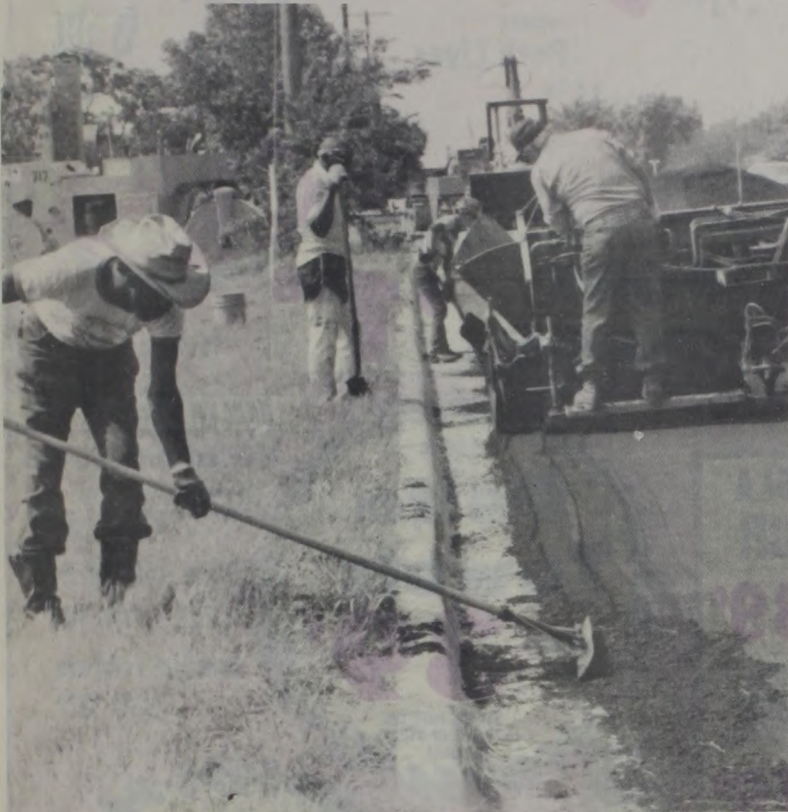
Another Muenster street gets the benefit of an improved surface as this machine applies a layer of ready mix. Staff Photo by Janie Hartman
