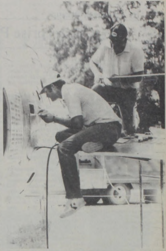
LEON WALTERSCHEID, left, and Adam Wolf, right, are replacing metal plates that once covered access doors to mechanical areas of the plane in City Park. Both men volunteered their time and talent, and both work at Weber Aircraft in Gainesville, who is supplying the materials for the repair work. It is hoped that with a couple more days of work the plane will be repaired by the July 4th holiday. Photo by Janie Hartman
