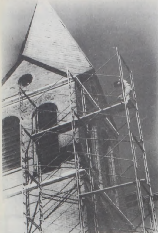
THIS SCAFFOLD IS BEING used in a roof repair project at St. Peter's Church in Lindsay. An outstanding feature of the roof will be copper on the steeple. In this photo a workman is securing planks after a few of them had been blown away in a mini storm. Photo by Janie Hartman
