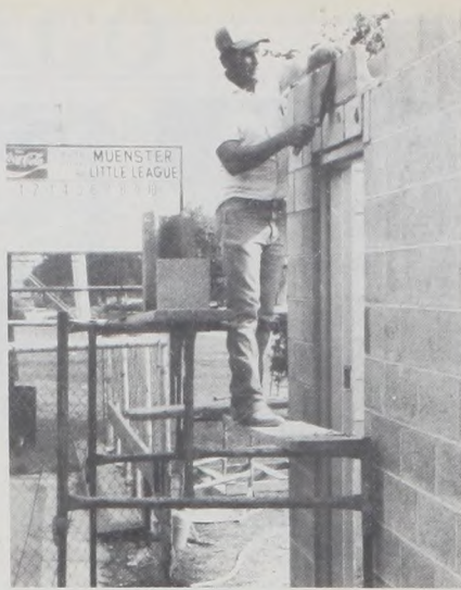
Progress at the city baseball park: Robert Klement is building the new Jaycee project, a rest room, beside the grandstand.
