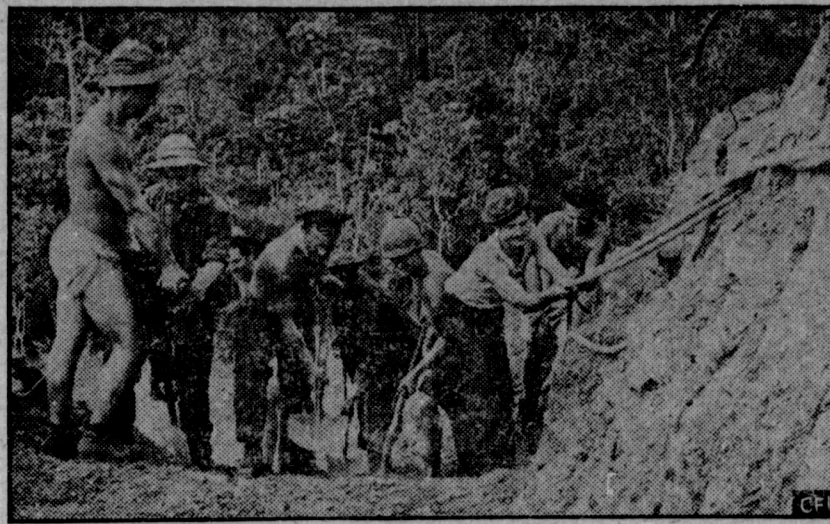
NEW GUINEA—(Passed by Army Censor)—American Army engineers are shown building "peep" road. The road is so steep that the men must hold on to ropes to keep from falling backward. Grade drops about 65 degrees behind them.
