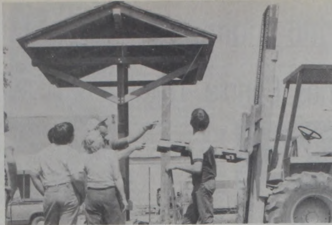
Rudy Koesler assisted by students from his MHS shop class, install a roof they built, on Mid-Park's recently completed park bench. Staff Photo
