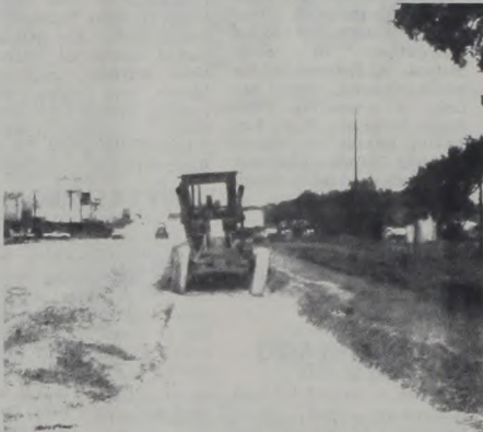
Construction of the 4-lane surface road to replace Muenster's former overpass is scheduled for completion near the end of August. Operation in progress here is mixing lime in a 6 inch layer of rock base.
