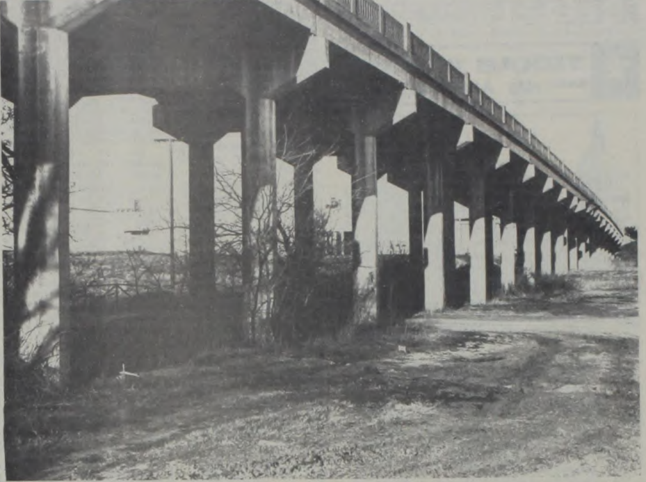
This Highway 82 overpass built in 1937 over the M. K. & T. railroad at Muenster, has been closed to traffic and will be replaced soon by a 4 lane surface road. The railroad tracks over which it was built was removed several years ago.
