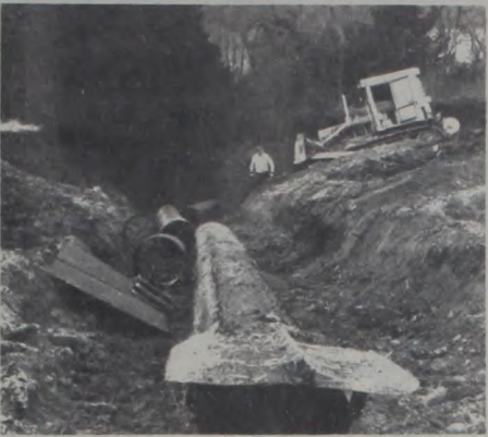
Grade stabilization structure being installed on David Brown farm. GSS will provide a safe outlet for water to be released free of large amounts of silt into Fannin Creek.
