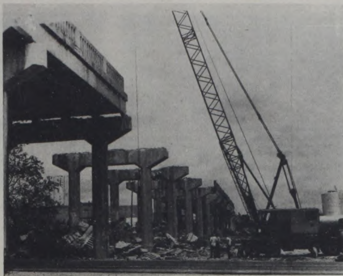
Demolition is under way on the overpass which was a landmark of Muenster since May 1937. The former two lane crossing over the MK&T railroad became obsolete when the railroad track was removed. The overpass has been replaced by a four-lane surface road. —Art's Photos
