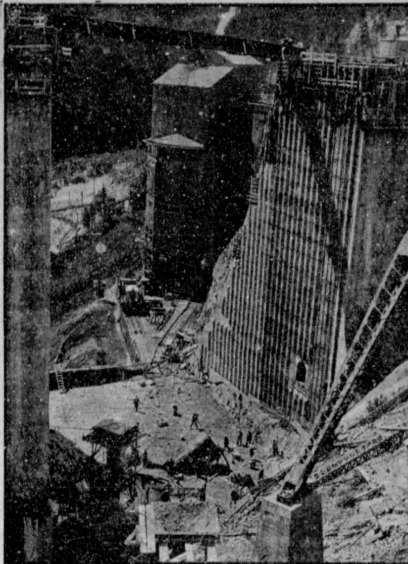
HIGH-SIDED HOLE —Only space left to fill in 564-foot-high Hungry Horse Dam, way up in western Montana, is block number 25 shown above. Two concrete pours will complete placement of all concrete used in the dam. Seen beyond the dam is the 139-foot-high concrete mixing plant. It turned out more than three million yards of cement for the dam, its power plant and other buildings used in construction of the dam which was built under direction of the Bureau of Reclamation, Department of the Interior. President Truman turned on the power Oct. 1 and dedicated the project which was completed 14 months ahead of schedule by the General Shea-Morrison Co. at a cost of $103,000,000.
