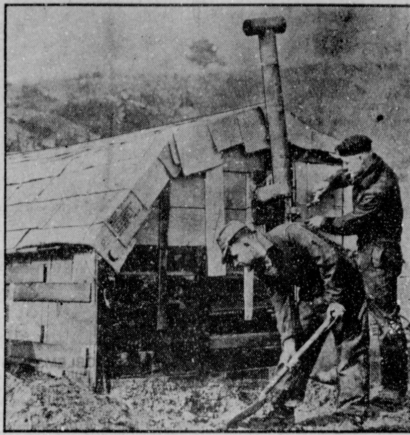
HOME OWNERS —A trifle displeased over the prospects of spending the rest of their Korean tours of duty in a fox-hole, these two enterprising Canadian soldiers built themselves this cozy cottage near the front lines. They are putting the finishing touches on the landscaping around their home built of ration boxes.
