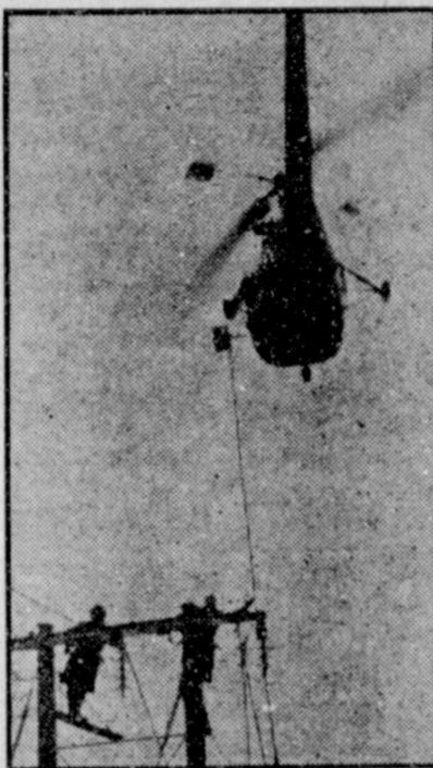
COPTER LINE LAYER —Hired by the Midlands Electricity Company, this helicopter hovers over one of two pylons at each end of a 1250-foot-wide valley near Malvern, England. The workmen reach out for a wire which will be used to haul a power cable line across the valley. Not only is the helicopter method a time-saver, but it is expected to avoid damage to hundreds of trees.
