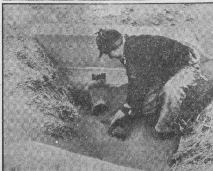
DUST STORM AFTERMATH —Albert Brabander digs out a culvert on his father's farm near Shawnee, Kan., after recent dust storms swept over the land. When the winds abated, loose soil like this was deposited like minor snowdrifts over many Midwestern farms, causing damage to crops which is still not fully estimated. Weather Bureau and Department of Agriculture officials admit that nature may be setting the stage for storms which could match the disastrous "Dust Bowl" days of the Thirties.
