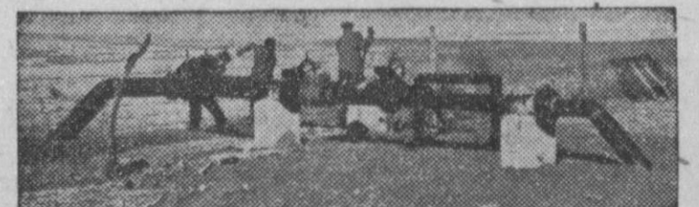
BEHIND GAS SERVICE there is something to build, paint, or repair every day, oftentimes in remote places. Above, a crew completes a control valve installation, part of a new compressor station. In the last three years, Lone Star has invested over $100 per customer to assure dependable service. Yet, you enjoy conveniences and comforts of natural gas service for a year around average of less than 15c a day.
