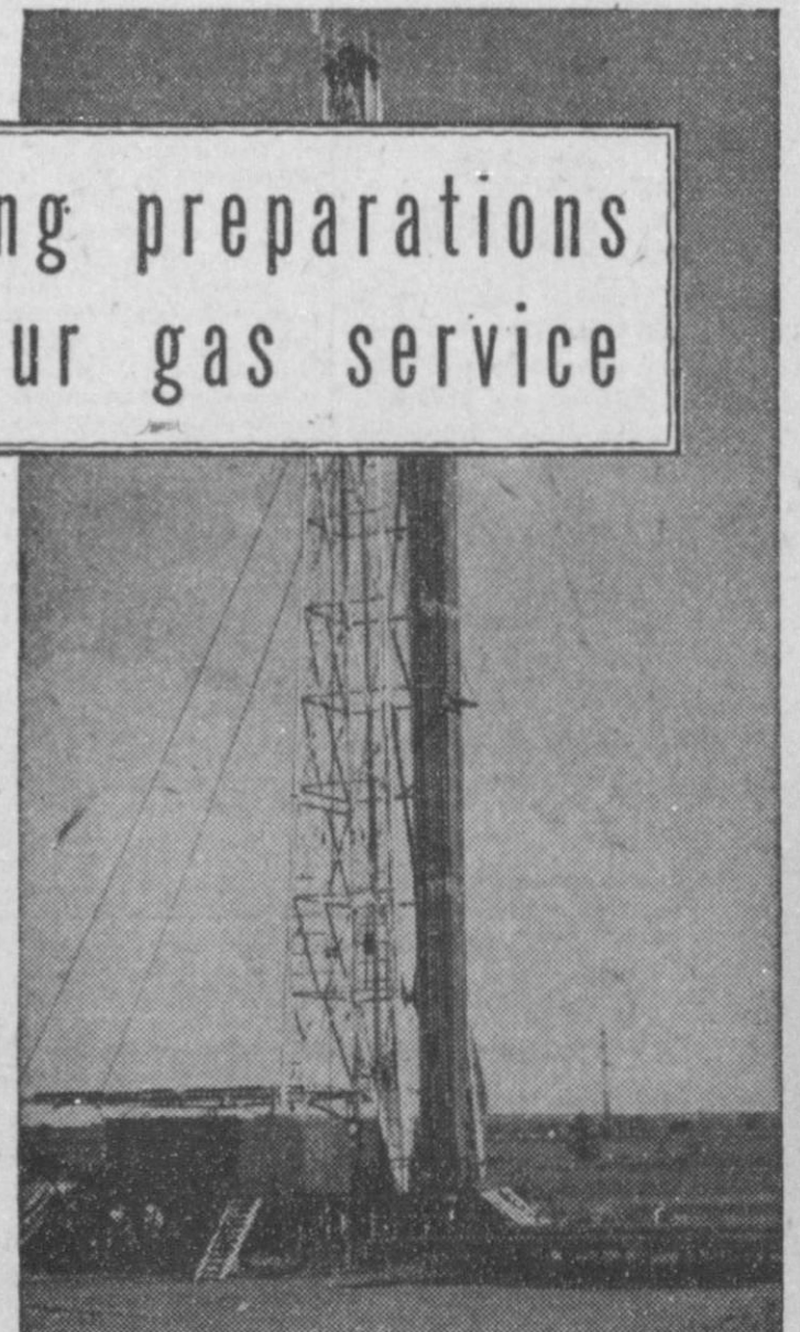
ROUND-THE-CLOCK drilling operations on this well were in their eighth week when this picture was taken. Months of painstaking work preceded the drilling. It has taken years of exploratory activity to obtain 1,140 wells (in over 100 gas-producing fields) that now supply you natural gas.
