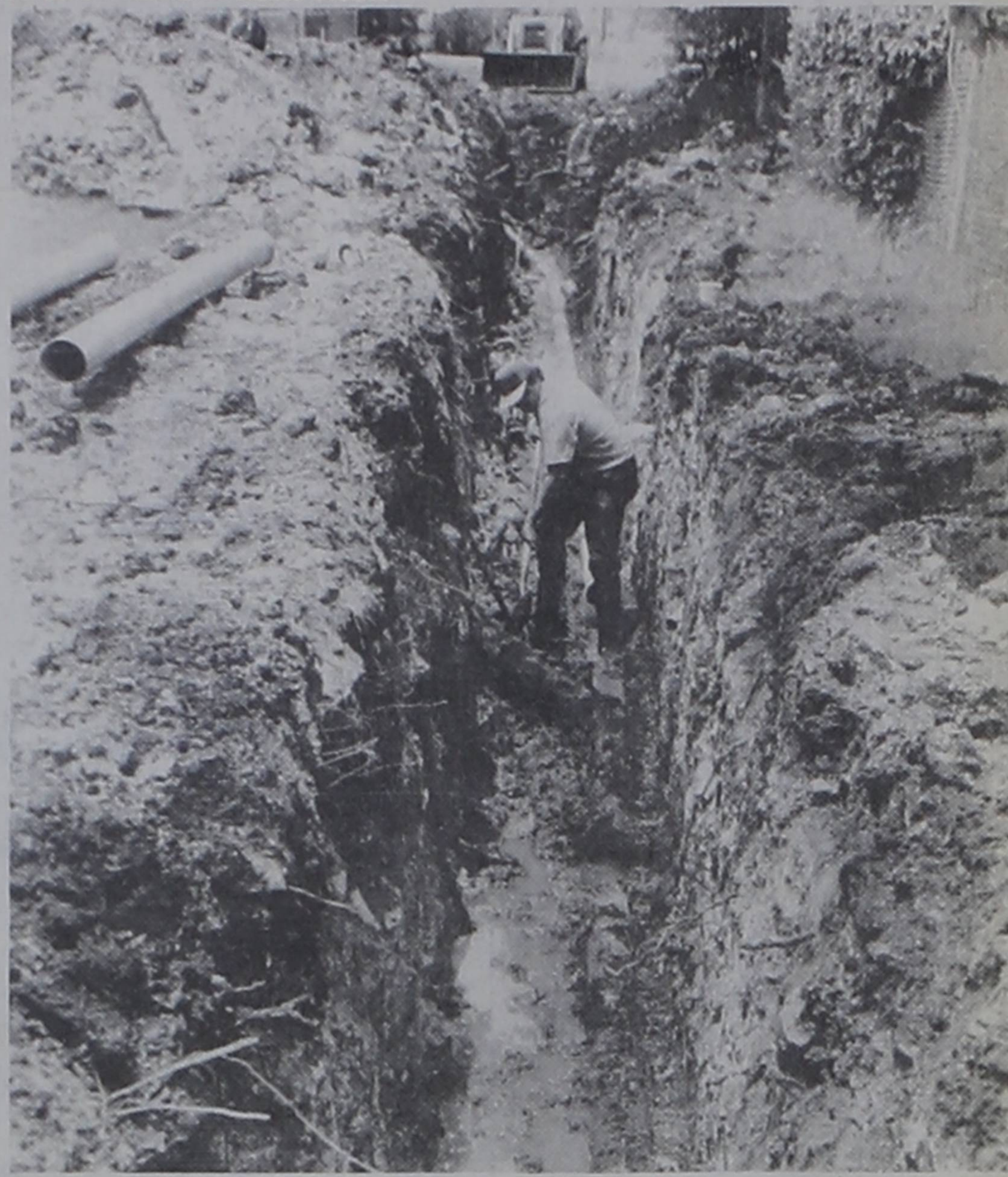
CHRIS YOSTEN , city employee, removes damaged sewer pipe in the alley of Block 18. One hundred and fifty feet of new line replaced the clay pipe that had been damaged by roots. Janie Hartman Photo
