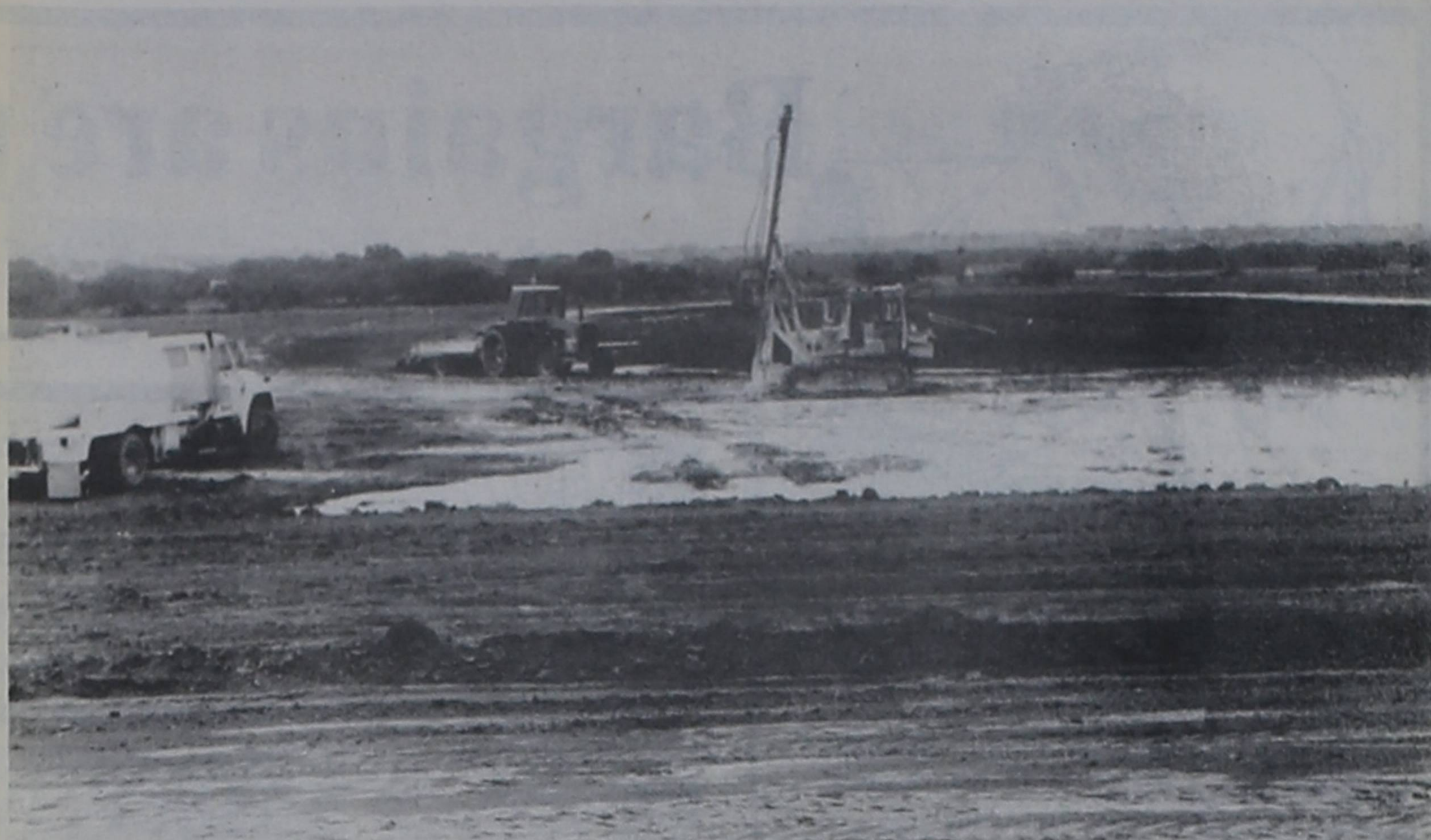
WORK CONTINUES on Lindsay ISD's new track and football field, as equipment shapes the ground and works the soil while weather permits.
