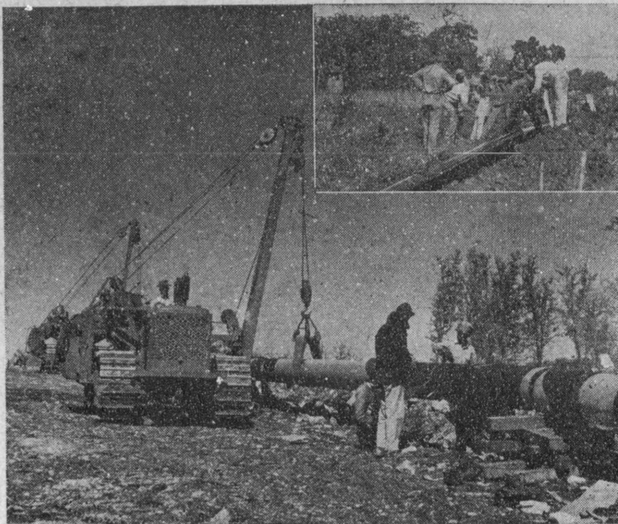
PROGRESS IN PIPELINING made great strides during Humble's history. It's a far cry from the back breaking hand labor (pictured at upper right) to the side boom tractor on today's spread. Humble's pipelines have
