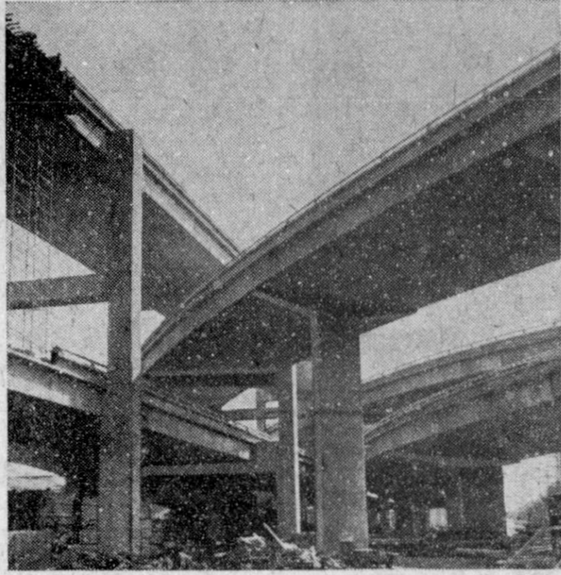
RAMP RENDEZVOUS — When it's finished, this complex system of highway ramps in San Francisco won't be the place to admire the scenery. However, the concrete complex is designed to smooth out traffic knots on the roads leading to the downtown section.
