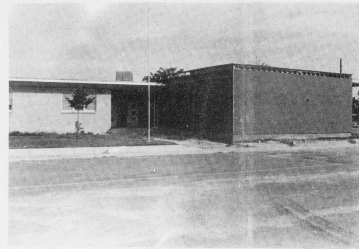
SCHOOL TAXES AT WORK ---Construction is continuing on the new Library at Dillman Elementary School. The library is just one of a number of improvements being made to the Muleshoe Schools. (Journal Photo)
