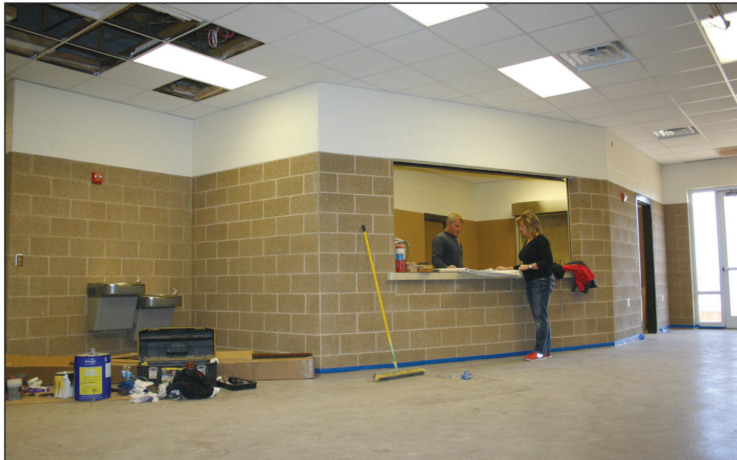
Sacred Heart Catholic School will soon get to enjoy the new concession stand which is part of the construction that began last summer. There is also weight and locker rooms to replace the fieldhouse destroyed in the June 2011 storm, and restrooms, coaches office, and storage. They anticipate that the addition should be finished in about two weeks. Shown studying the plans are Darell Walterscheid, left, and Janie Hartman photo
