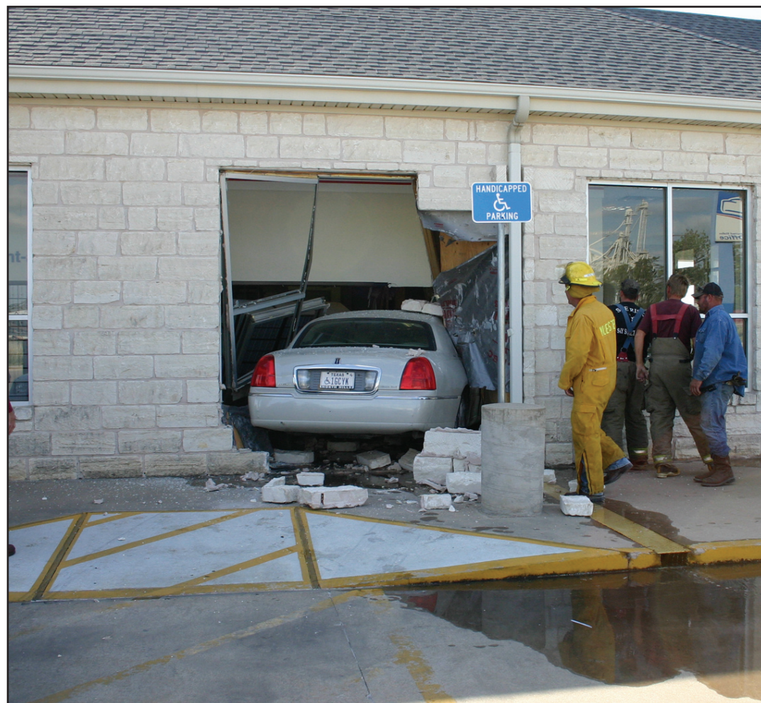
Late Tuesday afternoon, a gray 2007 Lincoln Town Car driven by Leonard Mize of Muenster crashed into the east side of the Muenster Post Office building. A report by Muenster Police Officer Tom Barr noted that the vehicle ran through the exterior wall and continued through an interior wall, coming to rest in the work room area inside. Mize continued to press the accelerator, causing the rear tires to spin until Leann Hacker, OIC of the Muenster Post Office, drew his attention and had him stop. The crash broke an overhead water line, flooding the area. There was extensive damage to the building and some mail boxes were damaged. See picture on page 2. Janie Hartman photo
