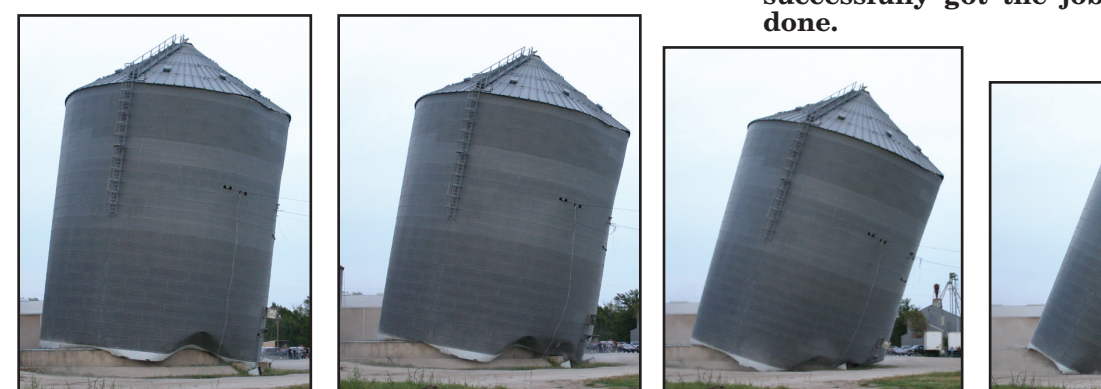
With dozers in place, what should have taken 30 seconds turned into hours to bring down a large tank at Muenster Milling. Above, workers replace busted cable with chain, only to have it tear through the structure. After all the professional suggestions to bring down the tank failed, good old fashion Muenster engineering successfully got the job done.
