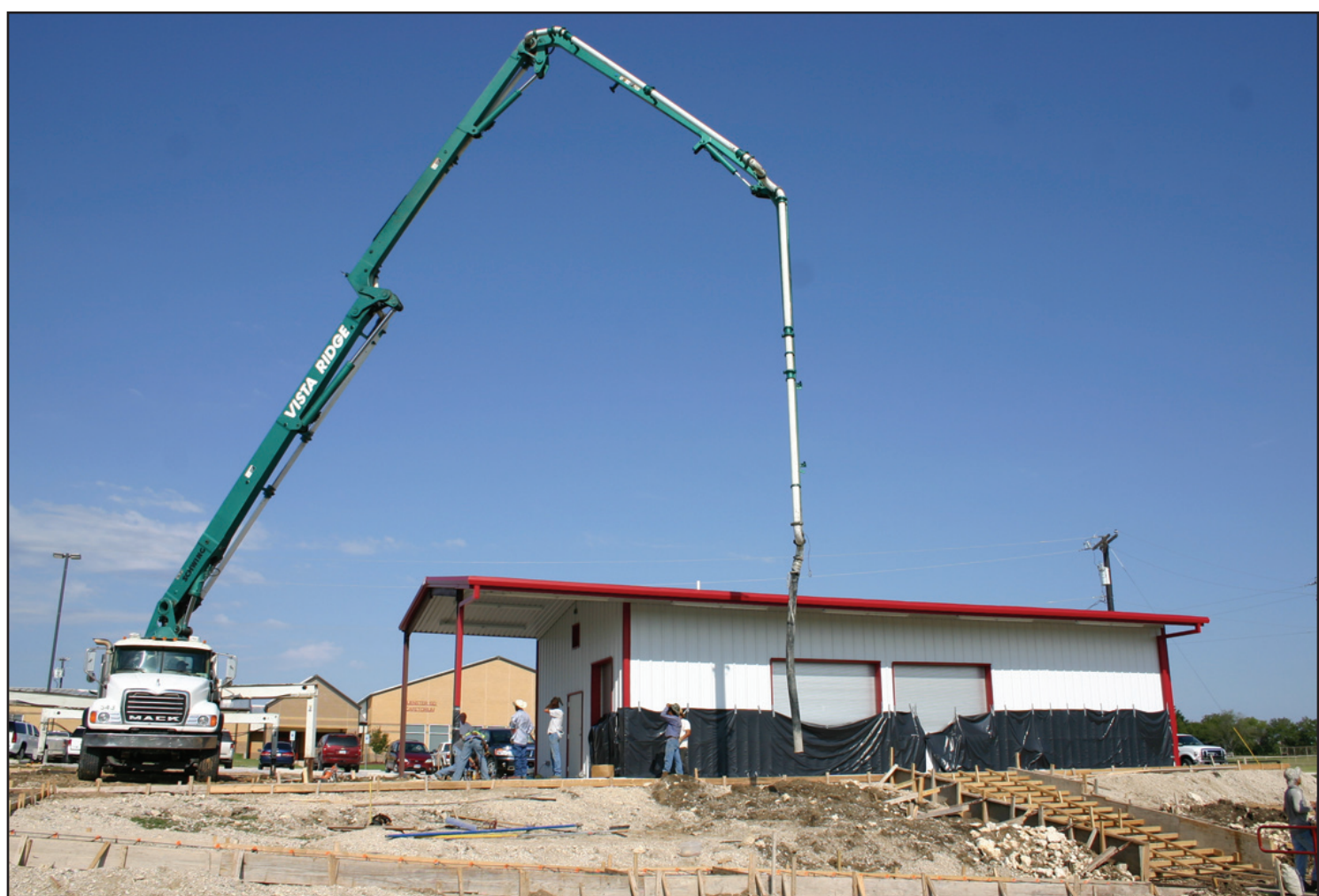
Work crews wait on the cement trucks to arrive to pour the walkway areas around Hornet Stadium's new concession stand. All improvements to the athletic facility should be ready for Muenster's first varsity home game Sept. 14. Janie Hartman photo
