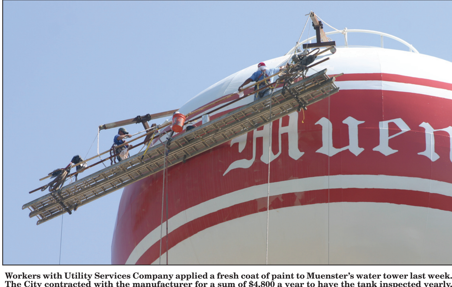
Workers with Utility Services Company applied a fresh coat of paint to Muenster's water tower last week. The City contracted with the manufacturer for a sum of $4,800 a year to have the tank inspected yearly, cleaned every two or three years, and painted every 10 years. The manufacturer sold its contract for the Muenster tower's upkeep to Utility Services Company of Warthen, Georgia. Janie Hartman photo
