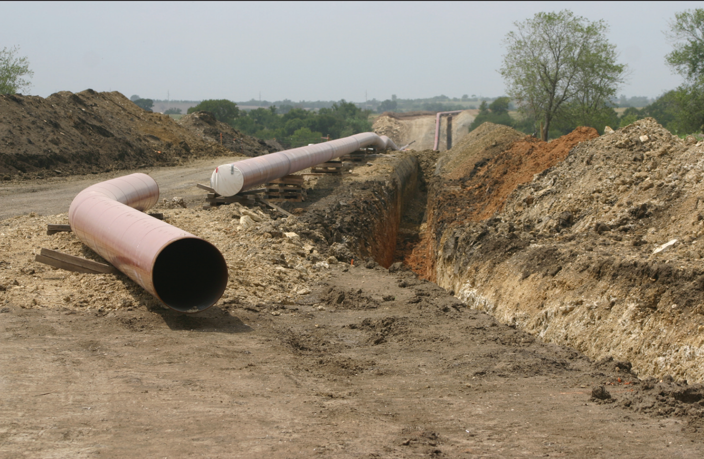
Construction continues on the Red River Gathering Line through Cooke County. The 95 mile natural gas pipeline will stretch from near Ardmore, Oklahoma to a Parker County processing facility, with its route mapped between Muenster and Lindsay. The picture above was taken looking south, where the line crosses under CR 438 east of Myra. The pipeline is scheduled to be operational by September. Janie Hartman photo
