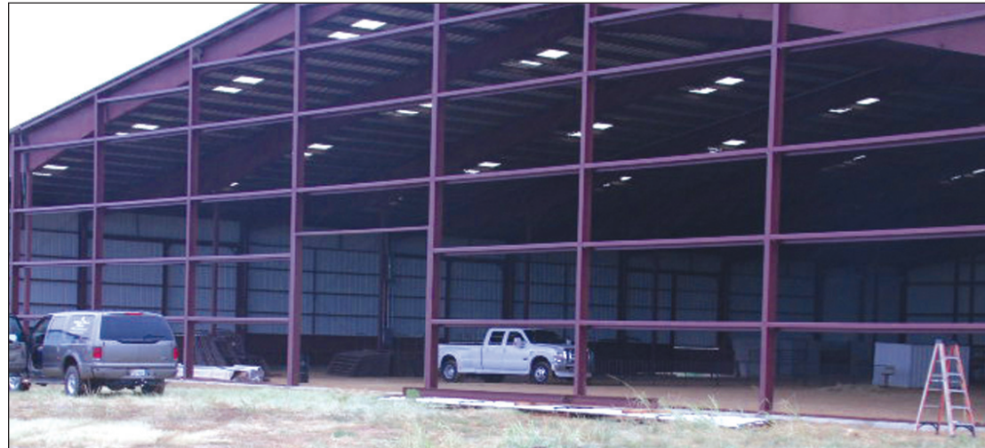
Closure of the south wall of the CCFA facility will allow better use of the building until funds are available to continue with the original design.
