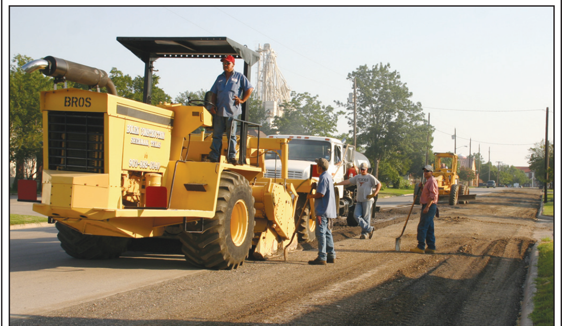
The road crew continued grinding up the asphalt and base on Oak Street this past week. Oak, from Hwy. 82 to 3rd, and 3rd Street from Main to Walnut will be getting a new surface, as well as patching around town. Janie Hartman photo
