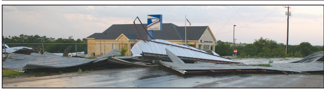
Metal debris from the Fisher Warehouse settled in the lot and street (East 2nd) near the post office. Janie Hartman photos
