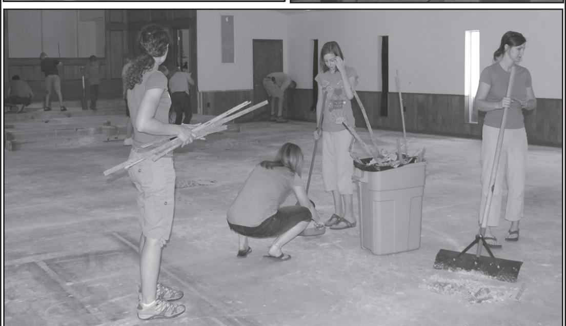
First Baptist Muenster has begun work to repair and renovate the sanctuary. Members joined together on Sunday, June 12 to enjoy a time of worship, food, fellowship, and prayer before rolling up their sleeves to begin clearing and preparing the sanctuary for work. The project is expected to be completed around Aug. 1, 2011. Pictured are, top left - Jay Johnson, Chris Watson; top right - Daniel Proffer, Tracie Bohl; bottom - Candice Watson, KaTina Johnson, Cassie Wright, and Jennifer Mills. First Baptist Church photo
