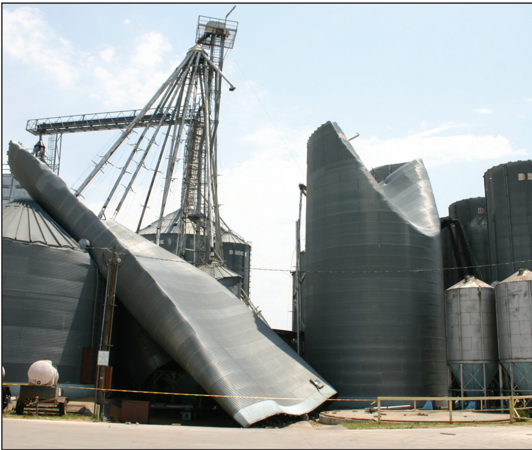
Collapsed Muenster Milling Company elevator tanks on South Main. Janie Hartman photo
