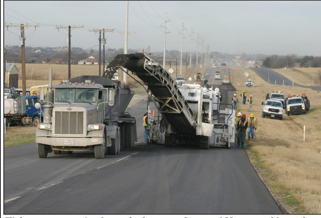
Highway construction began both east and west of Muenster this week as crews started tearing out the new surface placed last fall on Hwy. 82. According to the Texas Department of Transportation, specifications were not correct in that the mix was not dense enough, or compacted properly. The delay on the contractor redoing the job was that the hot mix season ended with the cold weather. It was noted that the job is being done at no cost to the State or the taxpayers.
