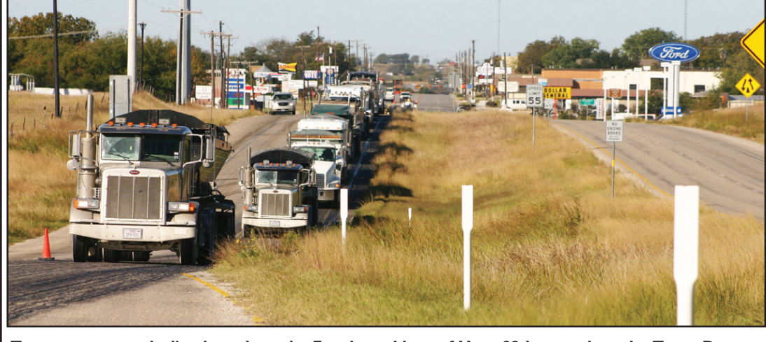
Twenty-some trucks lined up along the East bound lane of Hwy. 82 last week as the Texas Department of Transportation began a resurfacing project. Besides putting down a new lawyer going west out of town, the new pavement will go east to the FM 2739/CR 445 crossover. Showers delayed work, followed by the weekends. Janie Hartman photo
