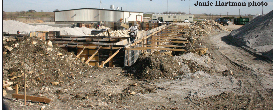
Workers take advantage of recent pleasant weather to construct the framework for the foundation of the new MISD practice gym. Janie Hartman photo
