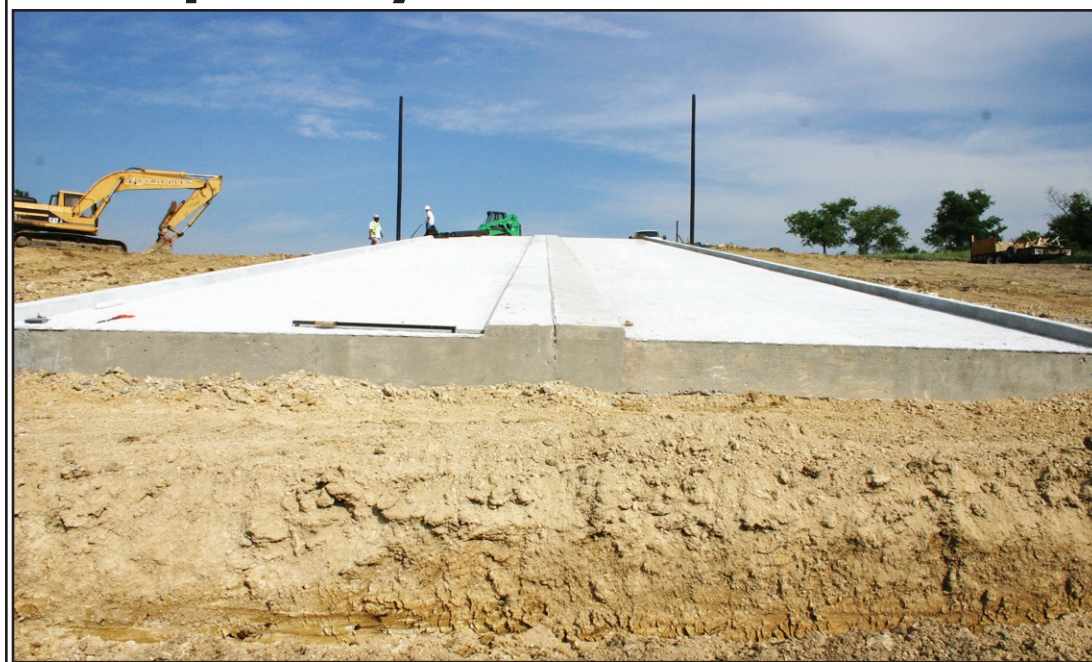
Muenster Lake's first-class boat ramp was completed last week and now waits for rain to refill the Lake for the pleasure of fishermen. Work continues on the parking lot area, including finishing the rip rap wall and fence installation.
