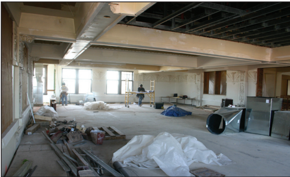
ABOVE - THE "UPSTAIRS" FLOOR BEING DISMANTLED. BELOW - GROUND FLOOR COURTROOM SHOWING FLOOR OF 2ND FLOOR ADDITION.
