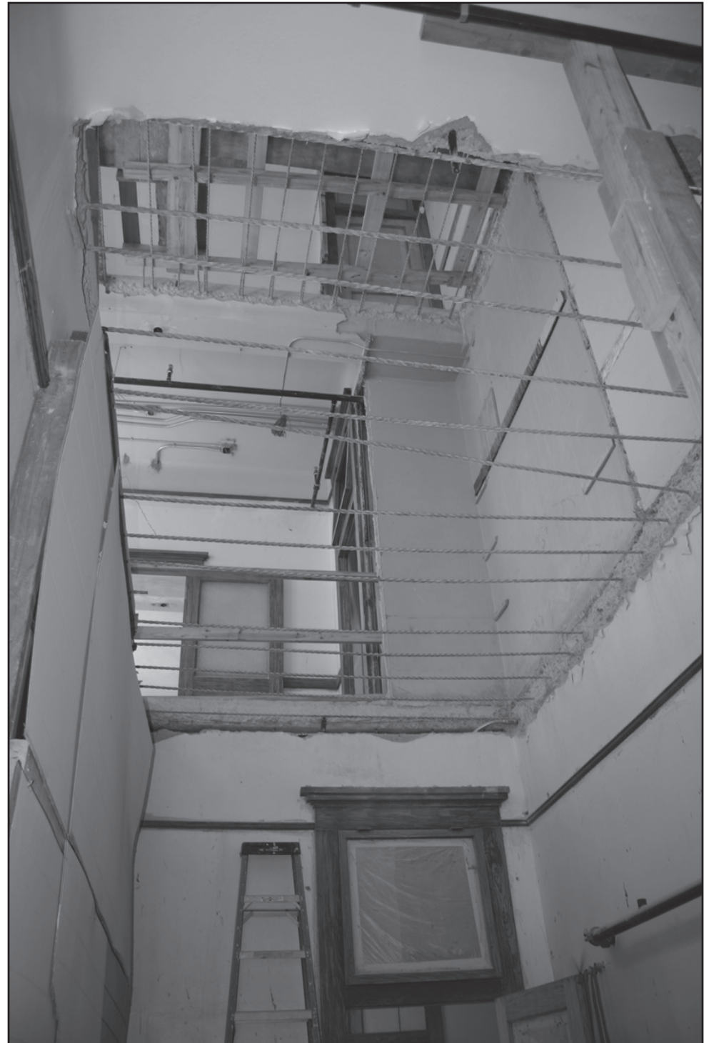
WITH THE REMOVAL OF THE FIRE ESCAPE SLIDE, A NEW ESCAPE ROUTE HAD TO BE INCLUDED IN THE PROJECT. PICTURED HERE IN MARCH 2010 - TEARING OUT FLOORS FOR THE NEW ESCAPE STAIRWAY.
