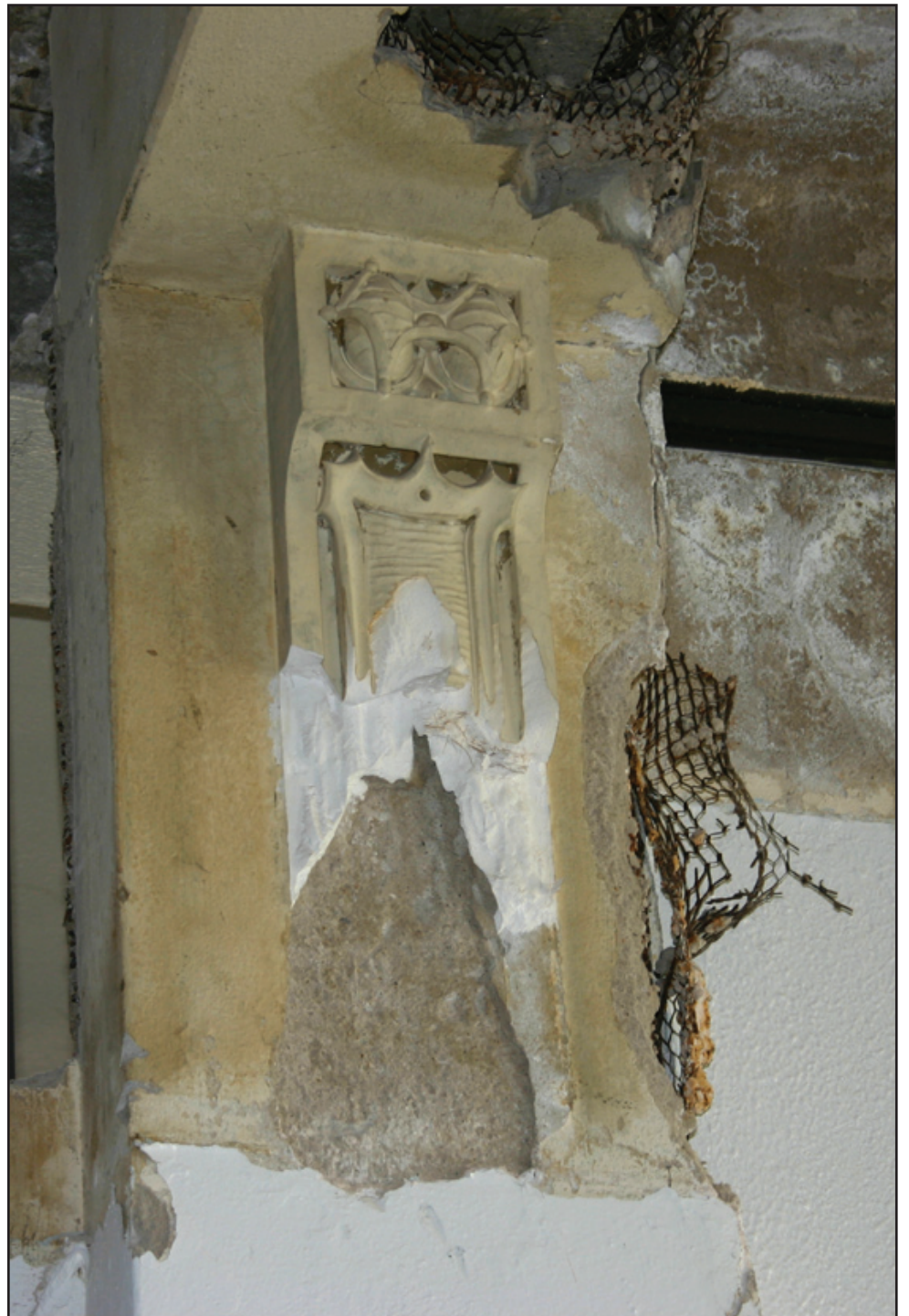
PLASTERED DESIGNER TRIM THAT WAS DAMAGED BY SLEDGE HAMMERS DURING EARLY REMODELING HAD TO HAVE CAST MADE FROM MATCHING PILLARS.
