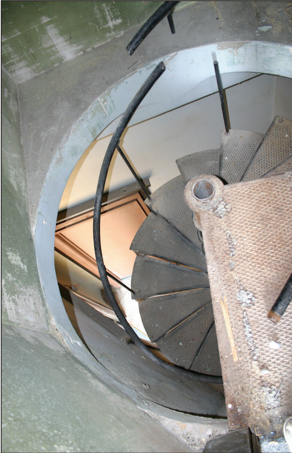
THE LONG ABANDONED SPIRAL STAIRCASE - THE BACK WAY USED TO BRING PRISONERS INTO THE COURTROOM.
