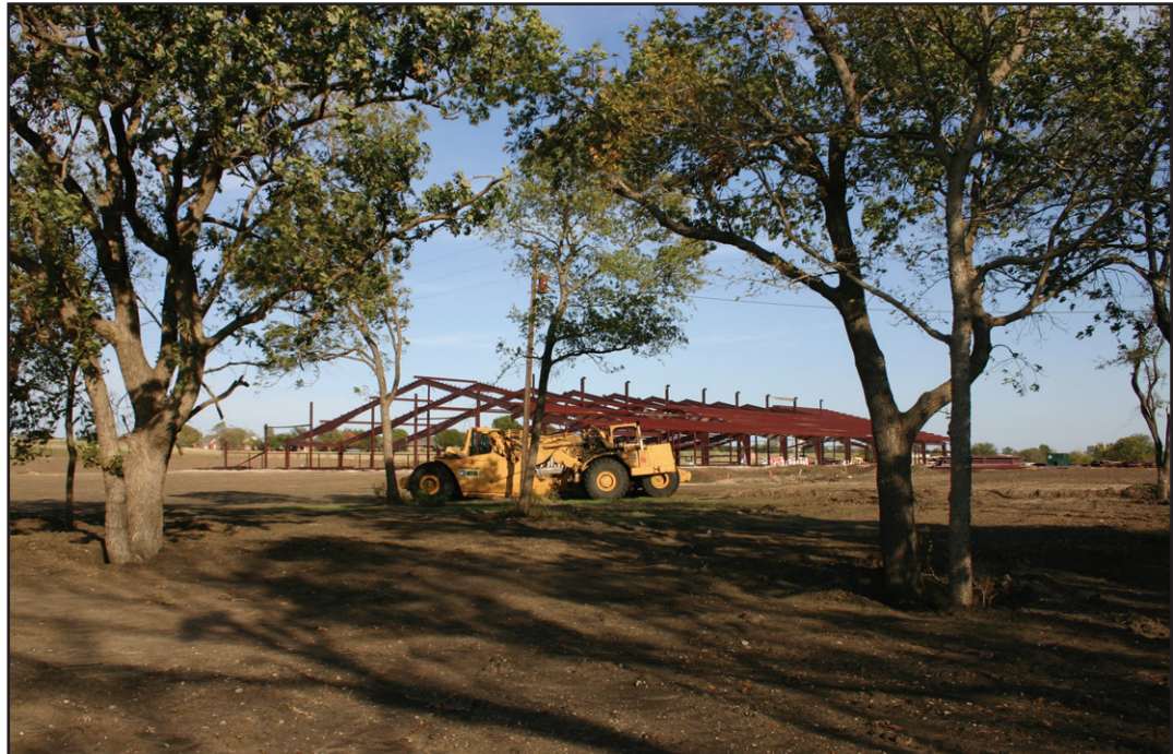
Going up - Germanfest, Inc. is becoming more than a drawing on paper, as the construction of the main building on the Germanfest grounds west of Muenster appears after months of dirt work. Janie Hartman photo
