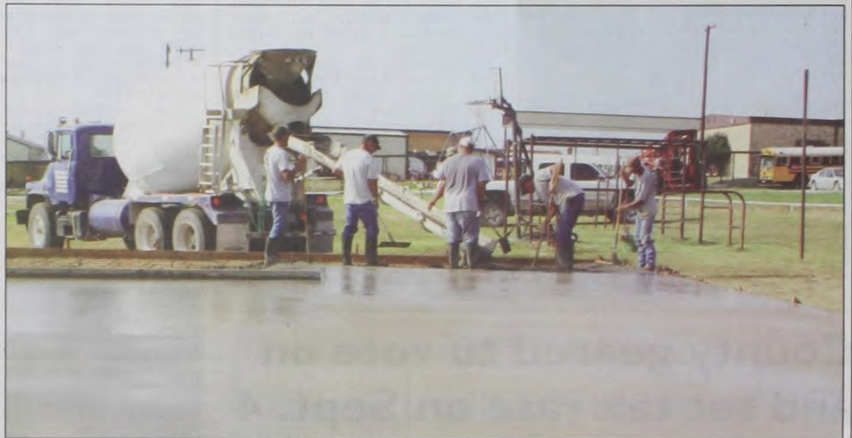
Dangelmayer Construction lays down a new basketball court on the playground at Muenster ISD Wednesday morning. The slab was built in the north playground/sports field area of the campus. Janie Hartman photo
