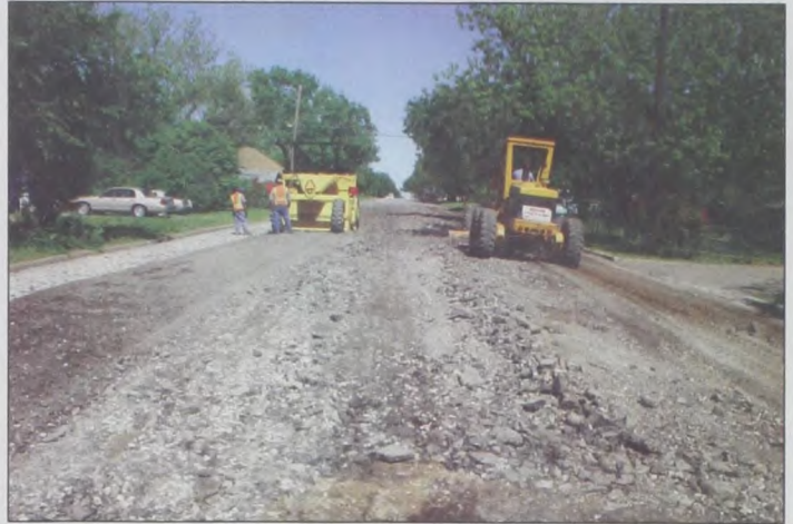
Several streets in Muenster are being repaired and replaced with a cement stabilized method of paving, covered with hot mix. Pictured is East 5th Street, between Main and Oak during last week's work. Janie Hartman photo
