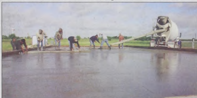
Dangelmayr Construction poured the flooring for the batting cage at the Muenster Jaycee Ball Park last week. The Jaycees are sponsoring a ball park benefit raffle on May 22. A $100 donation includes a party, with meal and beverages, and a chance to win lots of cash. Janie Hartman photo
