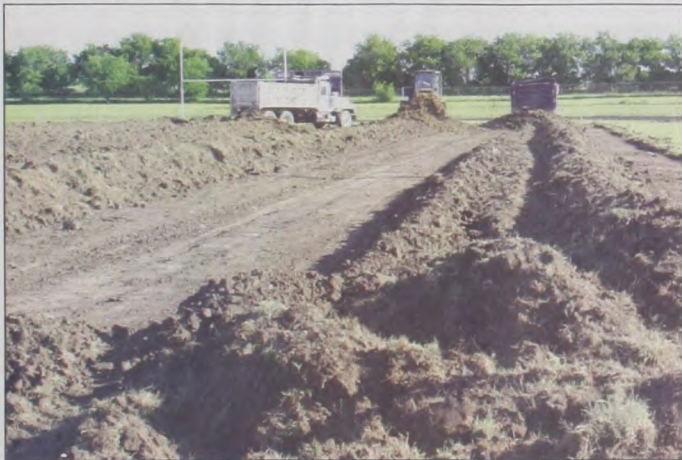
Dirt work is in full swing at Hornet Stadium, with G & H Backhoe removing the old soil as a first step toward building a new crown on the football field. Janie Hartman photo
