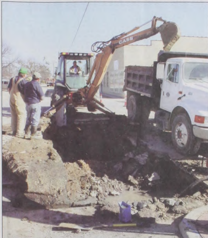
Freezing conditions earlier this week caused problems for City workers, including a busted water line on Main Street in front of Doc's. Police Chief Bob Stovall noticed water running down the street and notified City Hall. Workers took a day and a half to repair the line.
