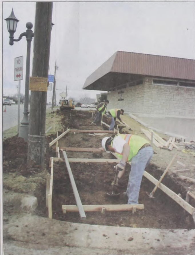
Work began this week on the latest Keep Muenster Beautiful landscape project, funded by the last Governor's Community Achievement Award earned by KMB. The concrete sidewalk, with brick pattern trim, will begin at the northeast corner of Division and Mesquite Streets, following Highway 82 west in front of the Telephone Museum, Nortex yard, The Center, and into First State Bank's frontage. KMB hopes to continue the project with future award money. Janie Hartman photo
