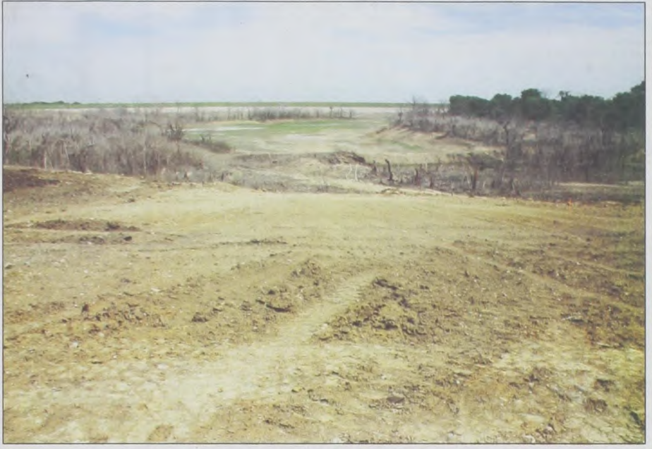
With drier weather, work has progressed in the construction of the boat ramp at Muenster Lake, located at the west access (CR 316) of the Lake. Shown is the "ramp" as it will descend into the water, ready for the concrete surface. Janie Hartman photo
